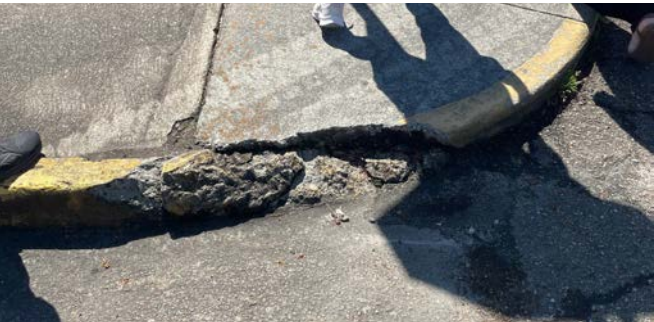
Sidewalk at the intersection of North and Dupree Streets that is broken and does not have an ADA-accessible curb cut. Image Source: Modern Mobility Partners, 2022
