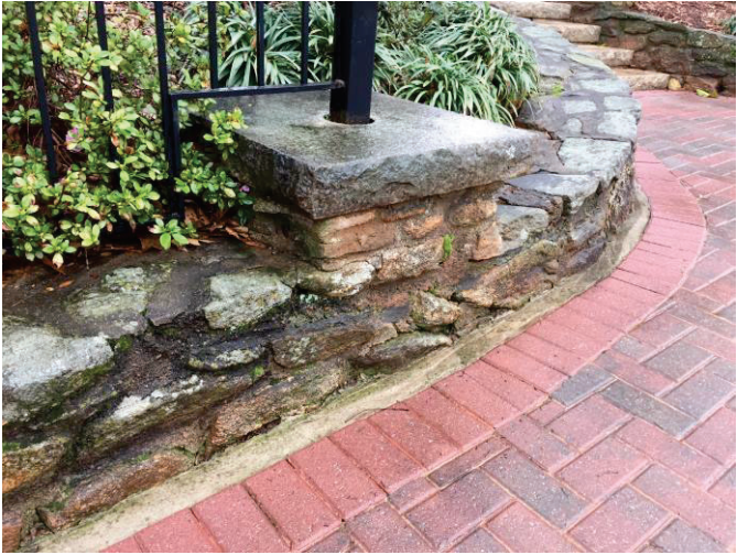
Stone seat wall & cut stone steps with red mixed beveled pavers at entry & walkways
