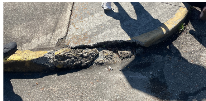
Sidewalk at the intersection of North and Dupree Streets that is broken and does not have an ADA-accessible curb cut.
