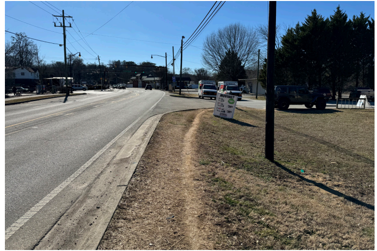
Worn foot path on west side of bridge
